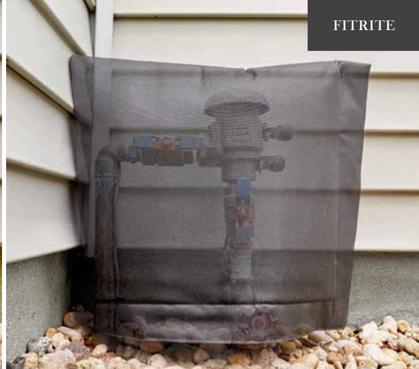
BACKFLOW ASSEMBLY WITH COVER
