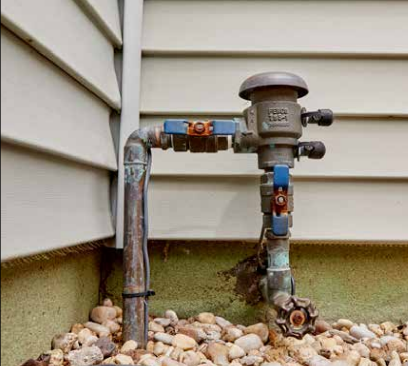
SPRINKLER SYSTEM BACKFLOW ASSEMBLY
